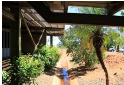
Storm water is directed into concrete gutters around the perimeter of the building
